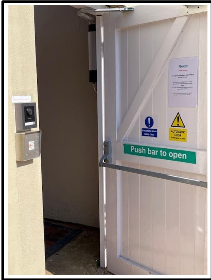
4. Automatic door opens outwards.
