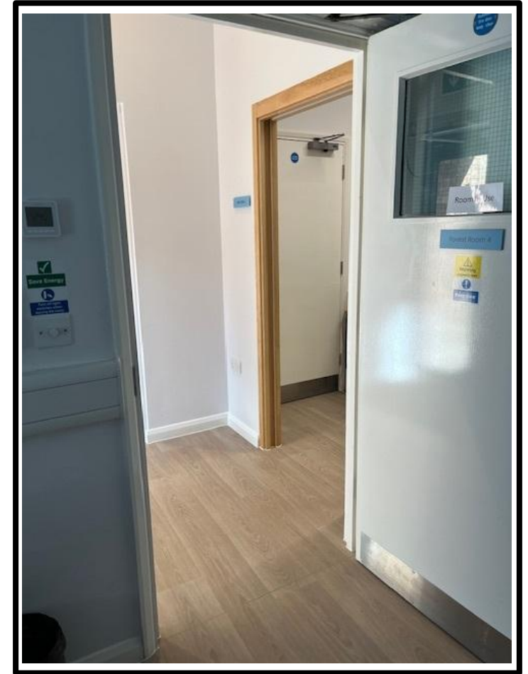
15. Enter/ Exit via automatic doors for easy access for all.
