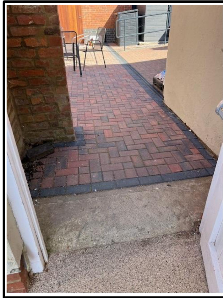
5. Entrance into garden – slight hump.
