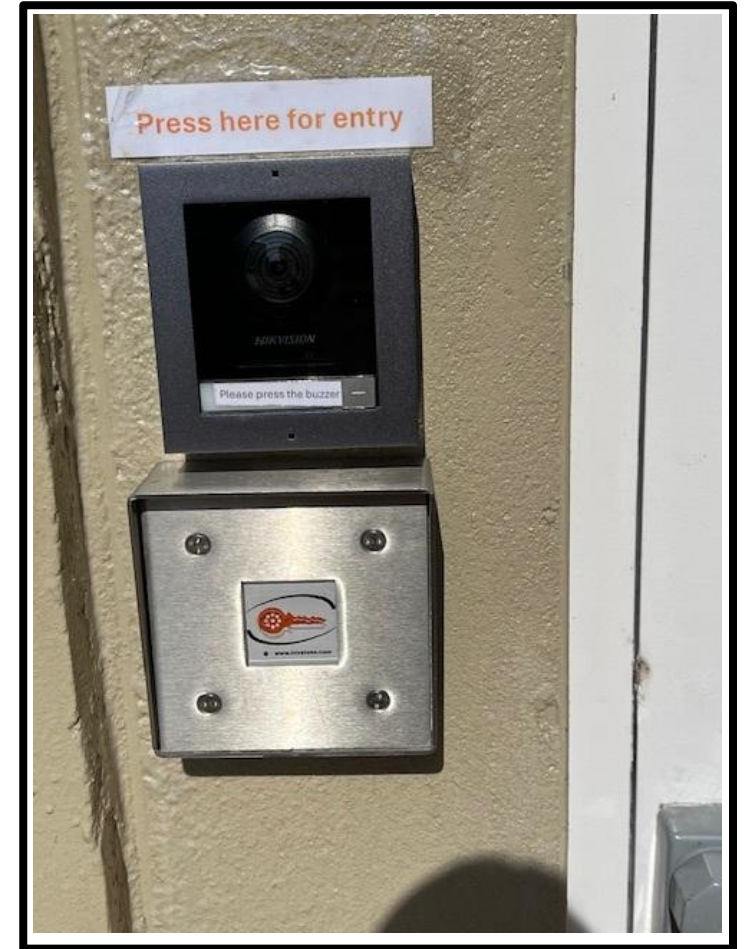
3. Press buzzer for entrance, automatic door opens outwards.
